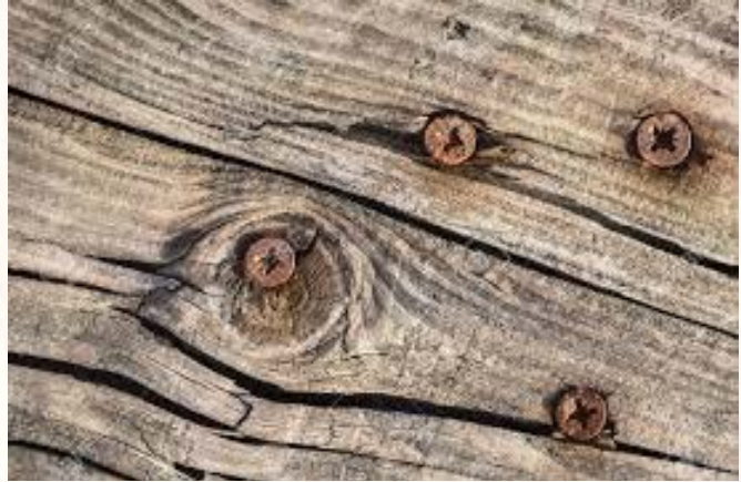
Figure 4: Example of “Nail Sickness” 图4、钉子疾病的例子
