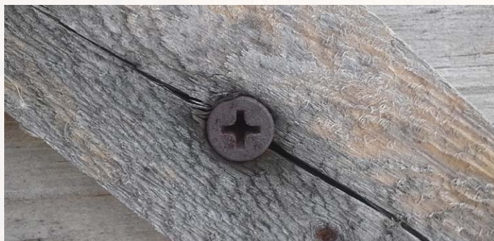
Figure 1: Zinc Plated Fastener Example in Alternate Treated Lumber After Several Years Exposure
