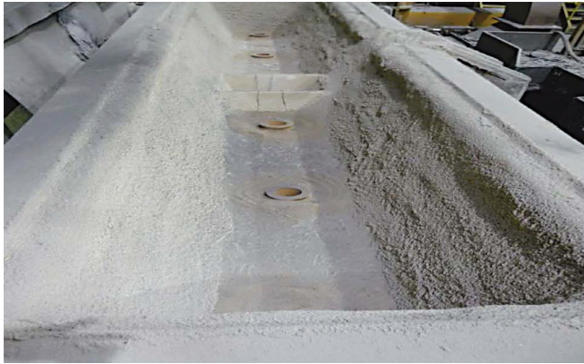
Fig. 3 — Inside view of the Tundish.
