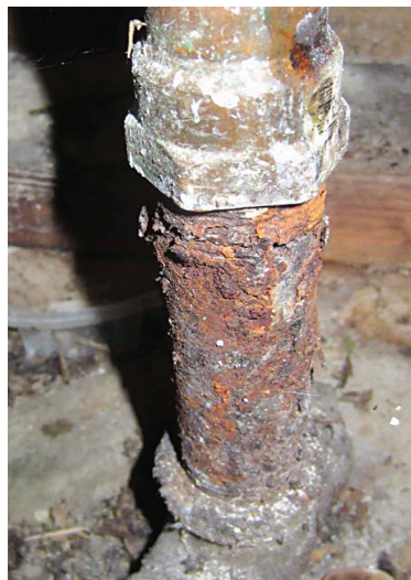
Fig. 1 — Copper fitting connected to steel pipe.
